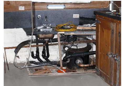
Sump pump problem behind bar fixed!
